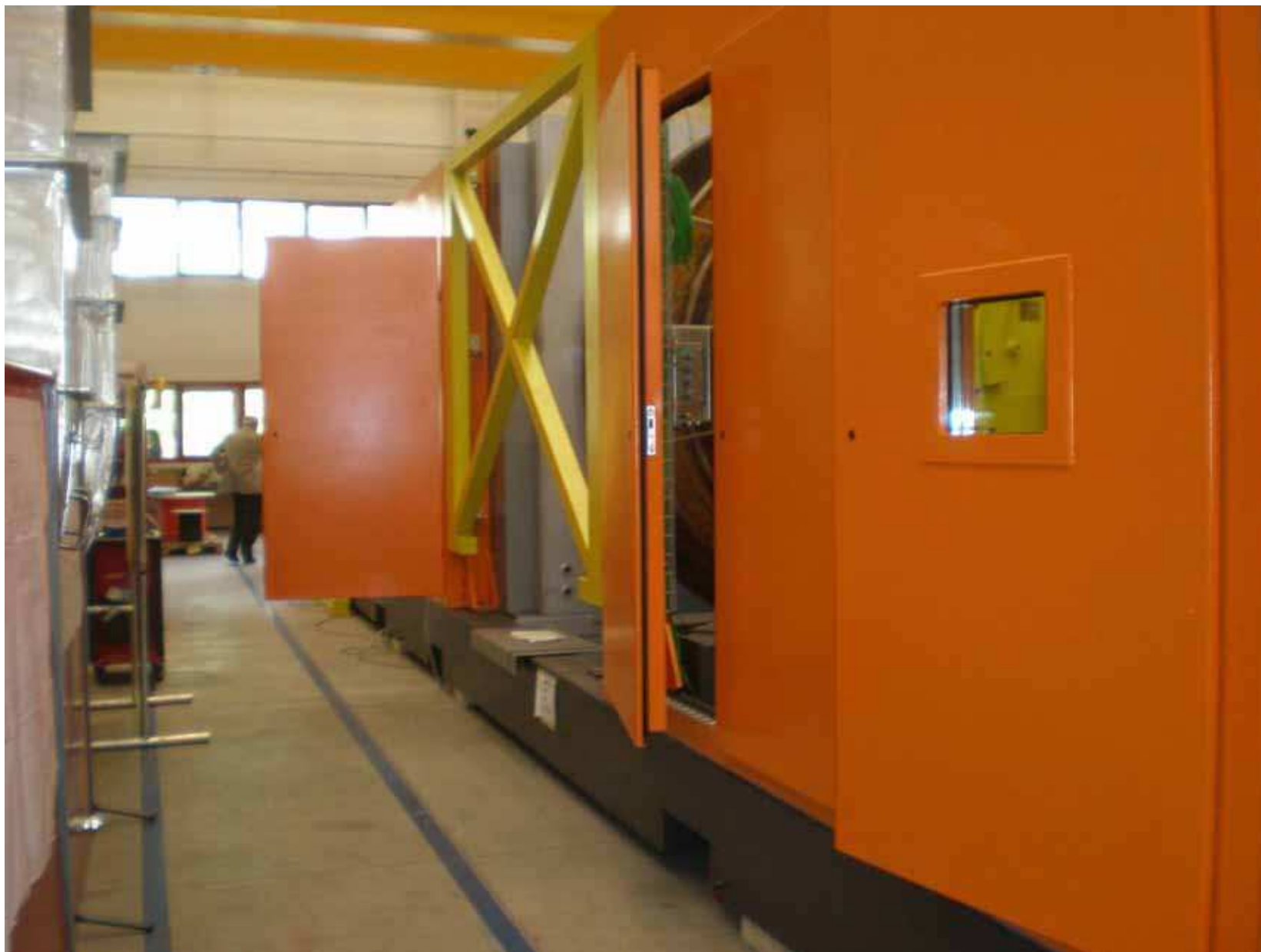
CCGT Imola ( turbina a gas )
